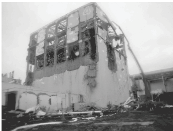
FIGURE 4.5 Damage to the structure surrounding Fukushima Daiichi reactor #4. (Photo courtesy of Tokyo Electric Power Co.)
