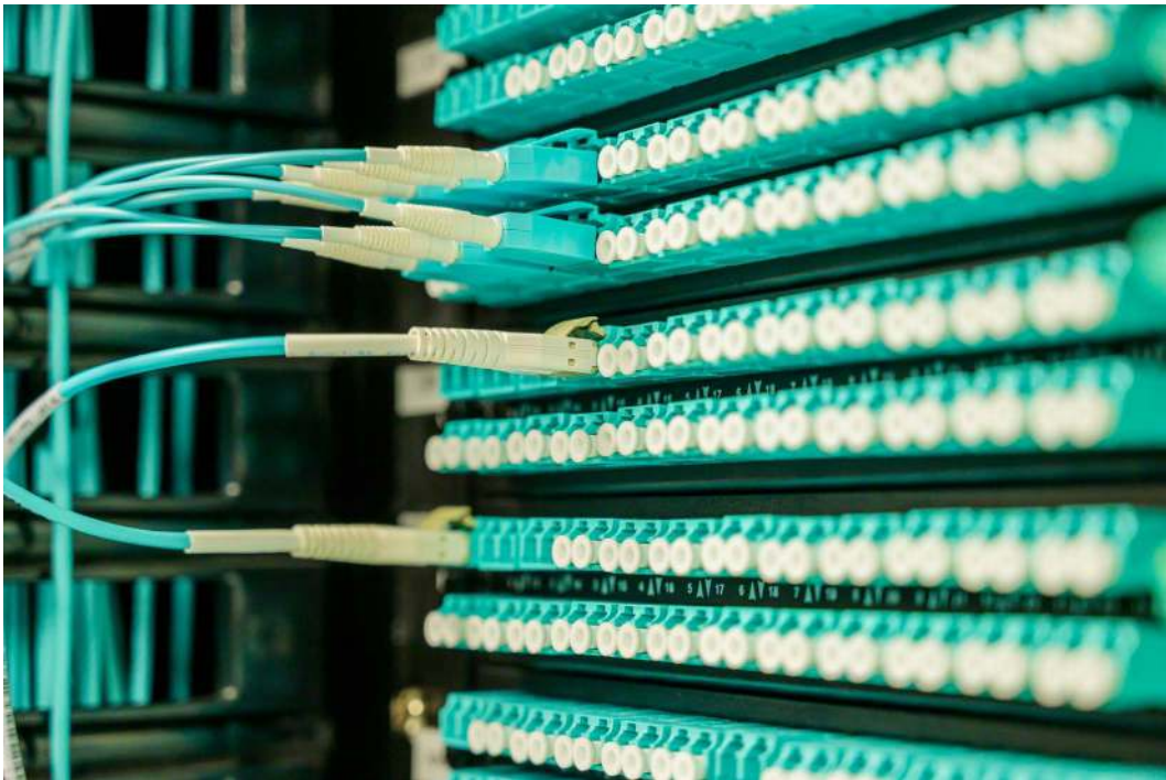
Figure 12.8: Fiber distribution panel
