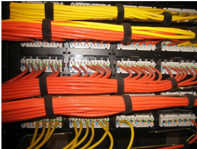
Figure 12.6: Rear of a patch panel
