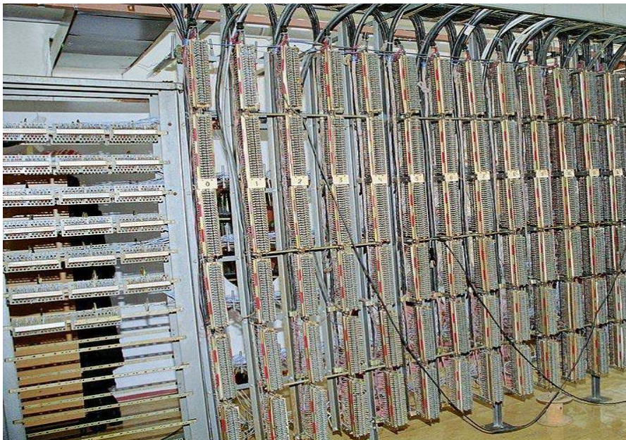
Figure 12.1: Main distribution frame
