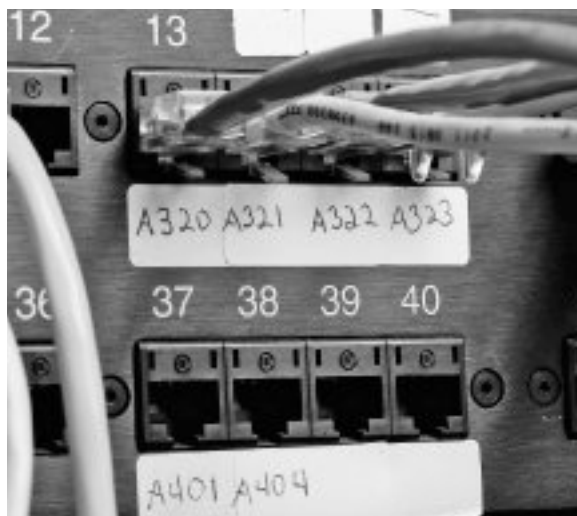
FIGURE 1.3-8 Typical patch panel in a server room
