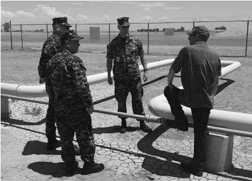
Major command—inspecting damaged fuel lines at Naval Air Facility in El Centro, CA
