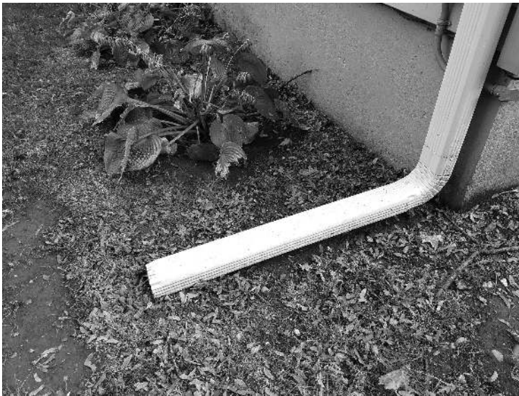
FIGURE 11.13 Long downspout to move water away from house.
