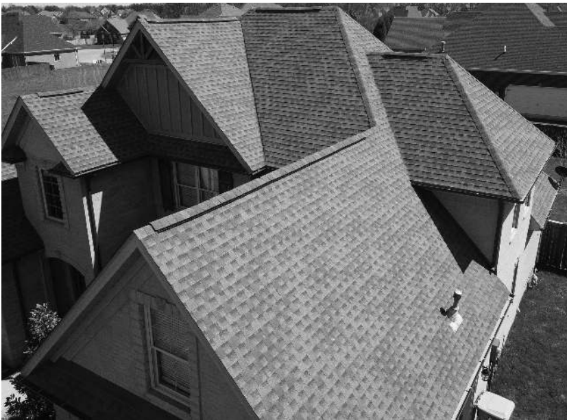
FIGURE 11.5 Roof valleys, which may overload gutters.
