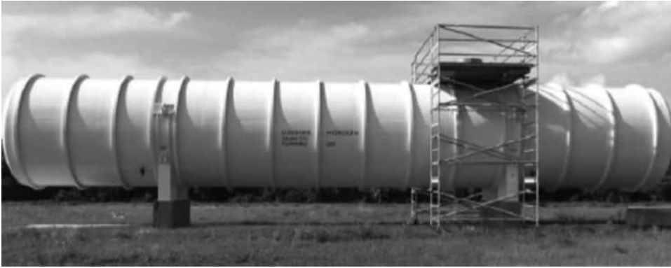
FIGURE 6.18 LH 2 storage tank of 125 m 3 with 80 layers MLI at the HTDF NASA KSC. Source: NASA
