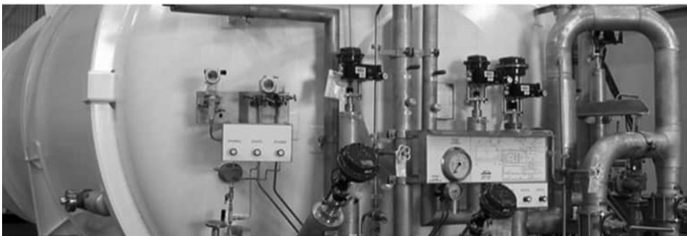
FIGURE 6.24 Upper: View of the 30-t liquid helium storage system at LHC Point 18. Lower: Side view of large LHe tank with gauges and valves for safety and controls [54]. Source: CERN
