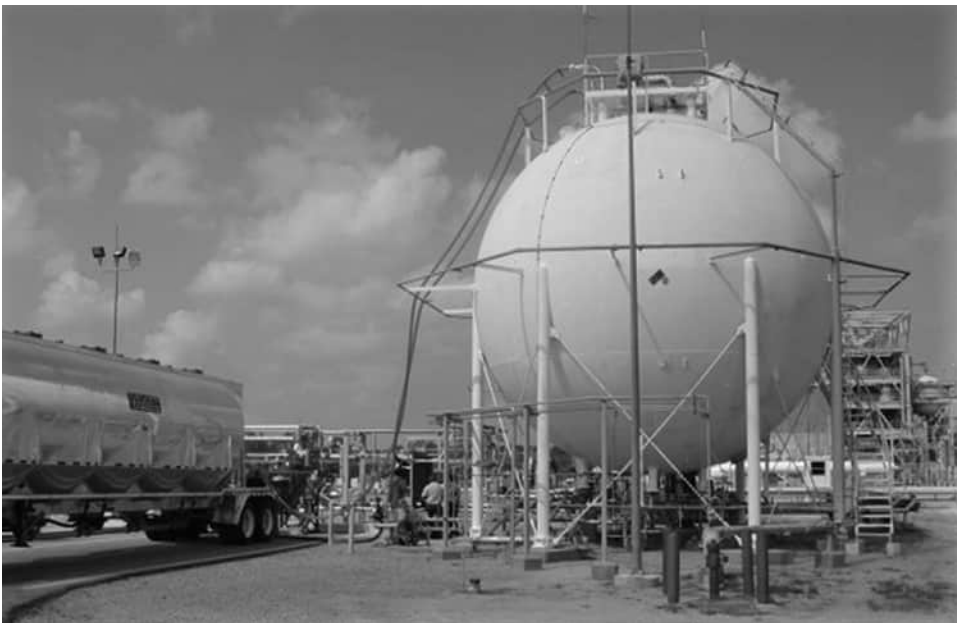
FIGURE 2.16 Field demonstration in a 190-m 3 LH 2 storage sphere at NASA Stennis Space Center. Shown is the process of loading glass bubbles into the annular space of the VJ tank.
