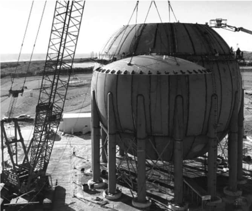
FIGURE 13.18 Construction of the world's largest LH 2 storage tank with a liquid capacity of 4,700 m 3 of at NASA Kennedy Space Center in 2020. Source: CB&I Storage Solutions, Photo Credit to McDermott International, Ltd.
