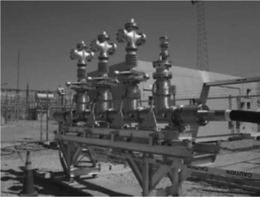
FIGURE 13.24 Field splice of a triaxial HTS cable and cryostat for the AEP Bixby project [29].
