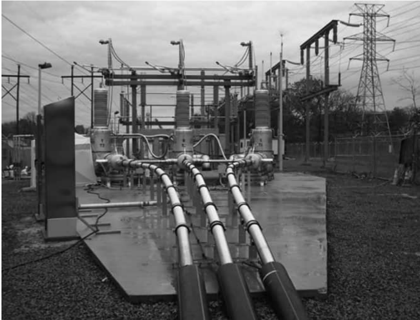
FIGURE 10.14 Long Island Power Authority—American Superconductor HTS cable terminations.
