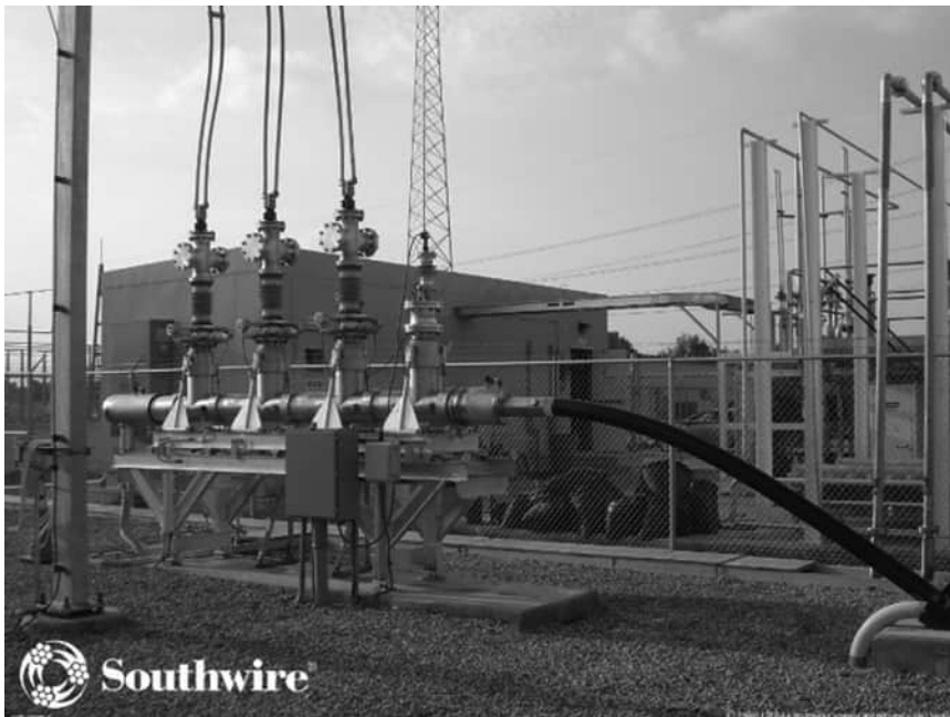
FIGURE 10.13 Termination containing the current leads for a high-temperature superconducting cable operating around 77 K.
