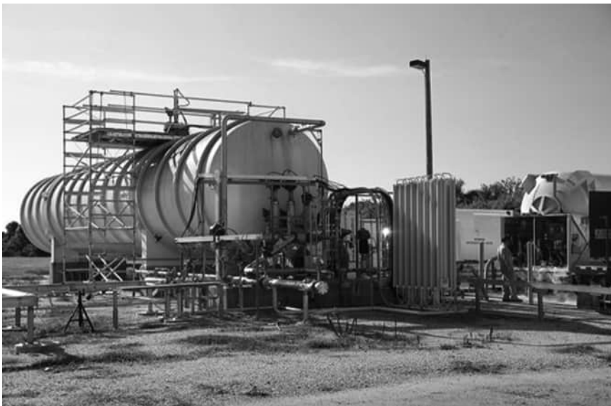
FIGURE 13.21 Field demonstration of liquid hydrogen densification and zero boiloff storage with a 125-m 3 storage tank and integrated helium refrigeration system at the NASA Kennedy Space Center's Cryogenics Test Laboratory. Source: Fesmire
