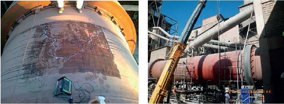
Figure 6. Impairment detection on the cement factory rotating furnace mantle via ultrasonic analysis [19].
