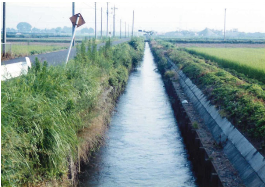
Fig. 10.2 Panoramic view at main drain 1 ( Photo by Akira Matsui ). Notes Photo date: July 2001. View from downstream to upstream
