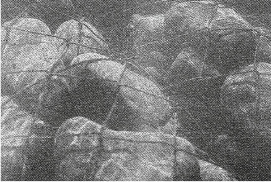
Fig. 2.10 Foot protection work. Source Reprinted from the Japan RiverFront research Center, http://www.rfc.or.jp/tp/files/02-03.pdf , Accessed October 30, 2021 (in Japanese)
