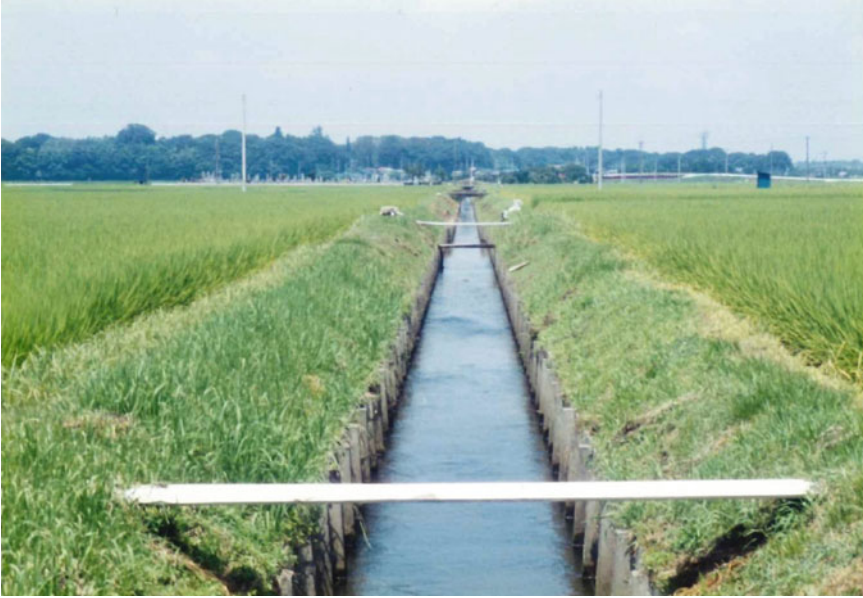
Fig. 10.4 Panoramic view at lateral drain 1 ( Photo by Akira Matsui). Notes Photo date: July 2001. View from downstream to upstream
