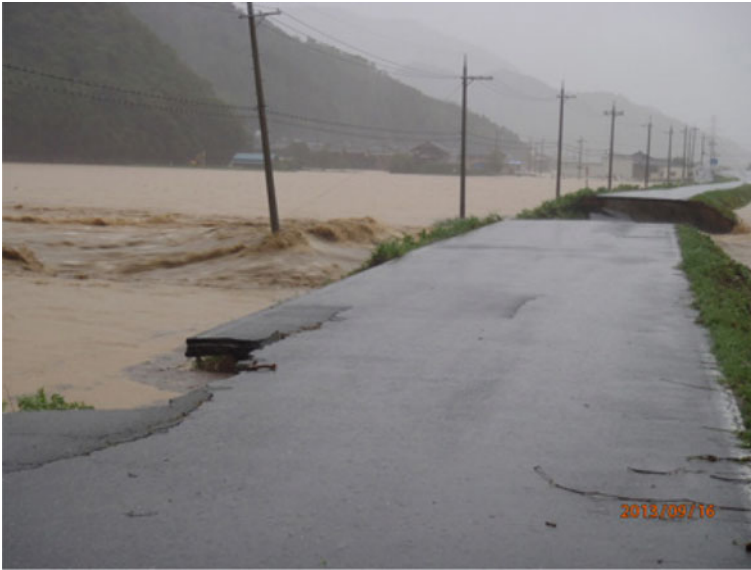
Fig. 7.6 Washout in the Nogi River. Source Reprinted from the Kinki Regional Development Bureau, Ministry of Land, Infrastructure, Transport and Tourism of Japan, https://www.kkr.mlit.go.jp/plan/saigairiburari/2013_t18/2013_t18_0043.html , Accessed October 31, 2021 (in Japanese)
