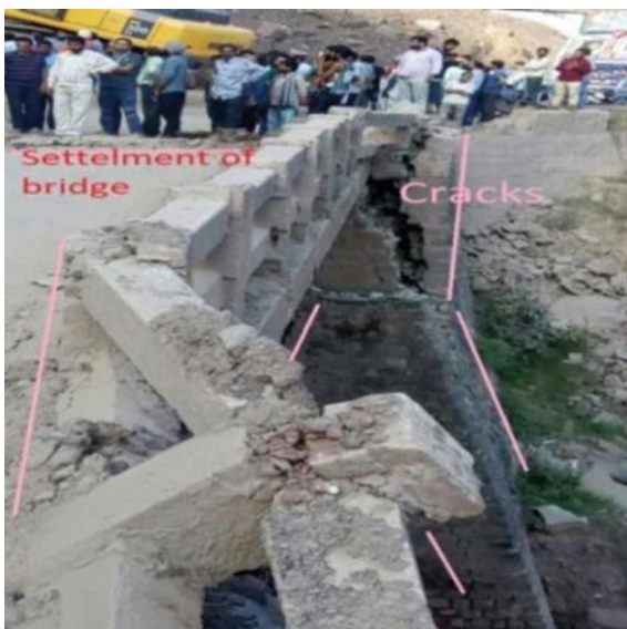
Photograph 6 Settlement of bridge and cracks in bridge abutment
