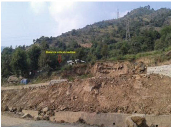
Photograph 7 House damage and geological strata near the ROW at Bali village
