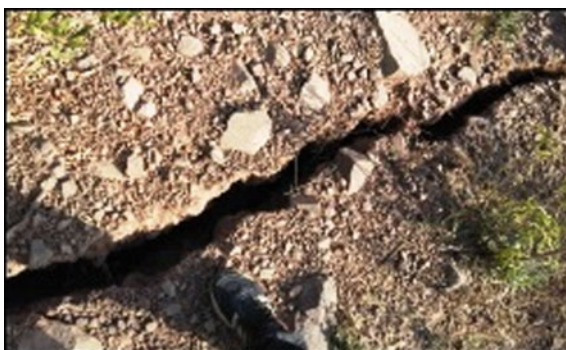
Photographs 5 Cracks developed at top of Samroli slide during September 2016 event
