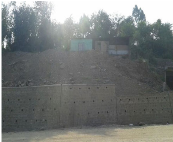
Photograph 10 House damage in critical condition and protection work at Todli village
