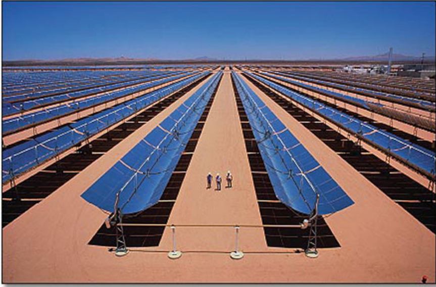
Fig. 8.1 A solar thermal power concentrator of parabolic trough type [4]
