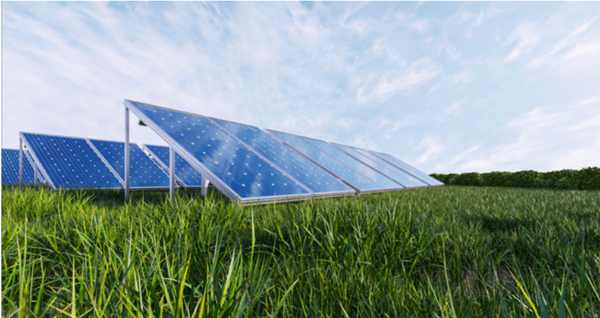
Fig. 4.2 Solar array for power generation
