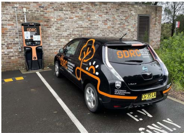
FIGURE 10.5 Electric car charging station.
