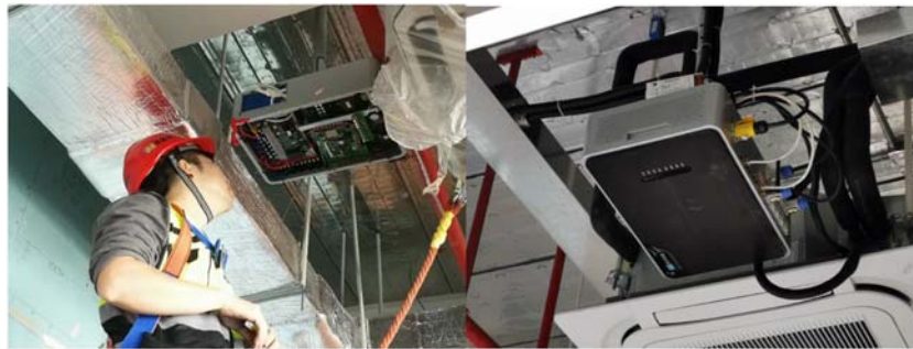
FIGURE 11.10 Commissioning of a smart DC/DC power converter box ( left ); and illustration of a DC power converter as installed ( right ).
