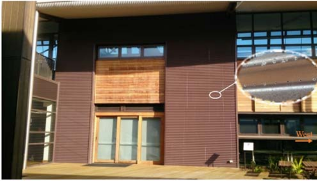
FIGURE 10.15 Illustration of the TSC system installed in the building.
