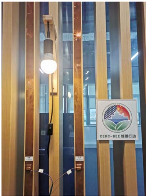
FIGURE 11.13 DC lighting with a 48 V DC naked copper bus bar.
