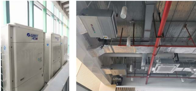
FIGURE 11.6 Outdoor units in the VRF ( left ), and fan coils and duct systems ( right ).
