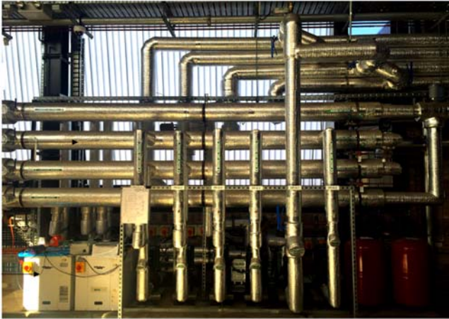
FIGURE 10.12 Ground source heat pumps and HVAC water distribution system.
