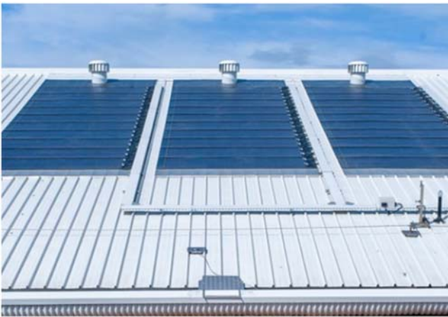
FIGURE 10.16 The rooftop PVT system installed in the building.
