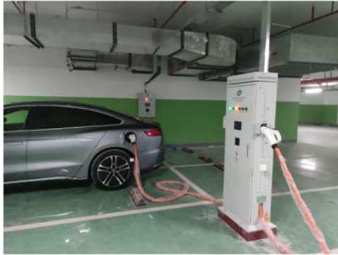
FIGURE 11.12 DC bidirectional EV chargers.
