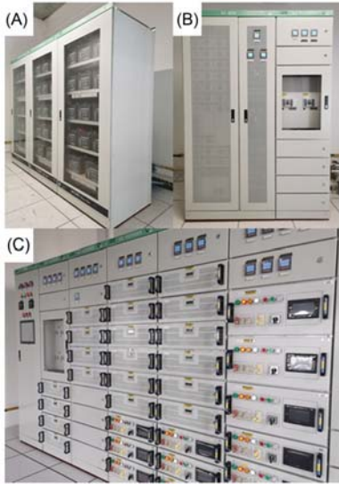
FIGURE 11.7 Controller cabinet for DC distribution: (A) battery storage, (B) AC-DC rectifier, and (C) power distribution controller.
