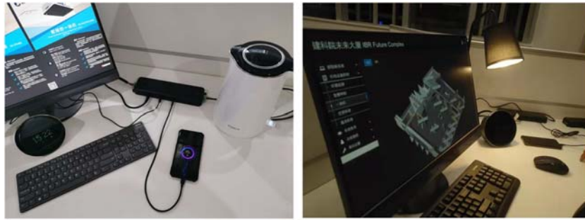
FIGURE 11.9 Low voltage DC socket to support multiple DC voltage levels for end-user devices.
