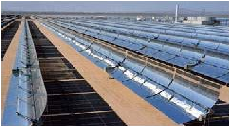
Figure 6. Parabolic Collector of the Power Plant.
