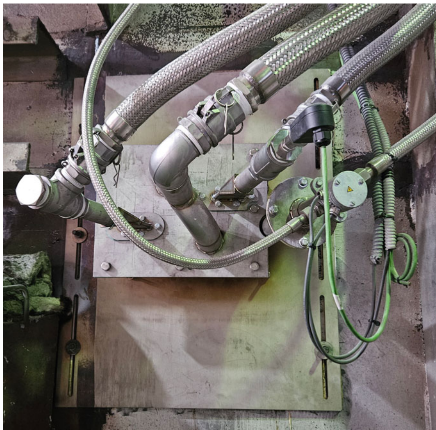
Fig. 4 HTHB mounted on a reverb furnace wall
