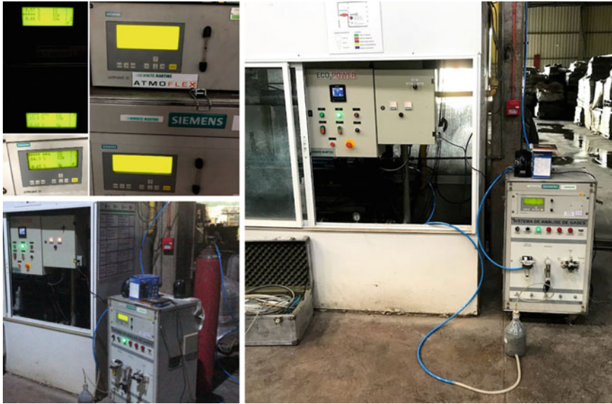
Fig. 6 Gas analyzer and combustion system’s electrical panel
