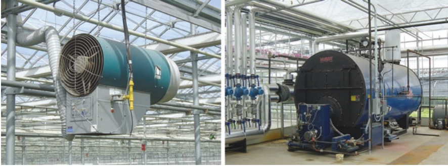
Fig. 11.1 Examples of a hot air (left; unit heater) and a hot water (right; boiler) heating system used in greenhouse operations. (Photographs by A.J. Both)
