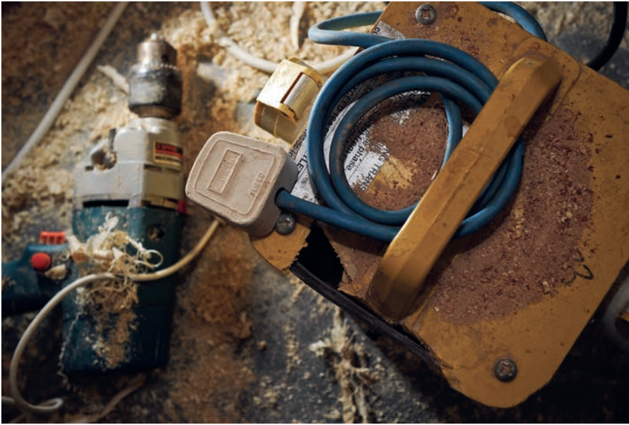
▲ Figure 7.4 Damaged transformer and poorly maintained equipment lead to a high risk of injury
