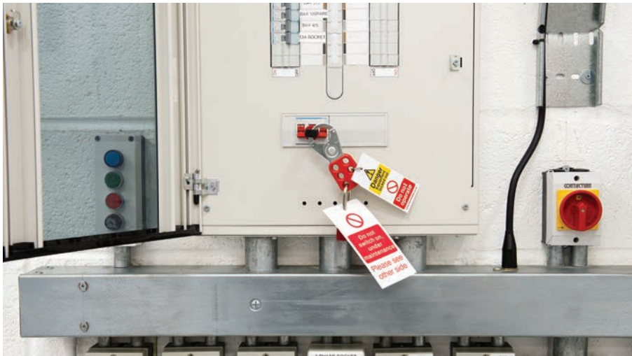
▲ Figure 7.13 Isolation of an installation should be part of a planned and agreed procedure
