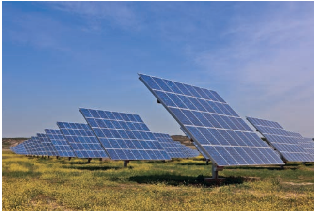
▲ Figure 1.26 Ground-mounted systems in a solar farm
