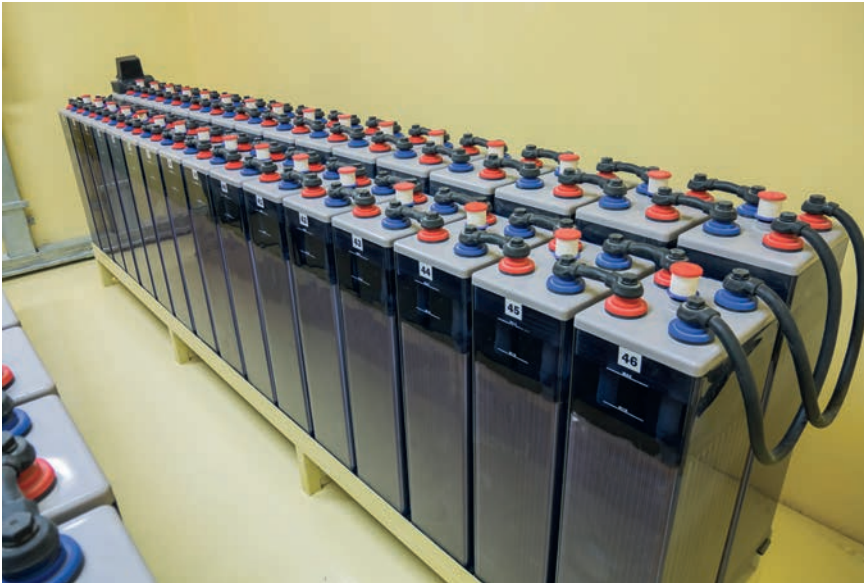
▲ Figure 7.11 Storage batteries
