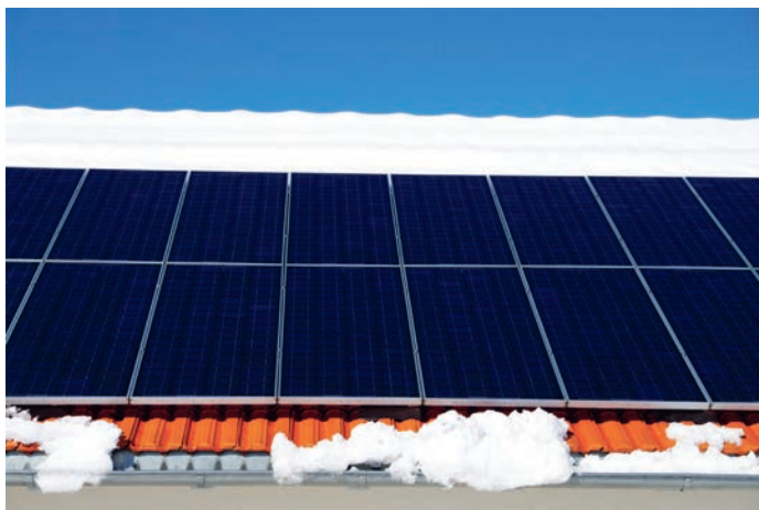
▲ Figure 1.25 Roof-mounted system
