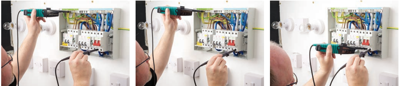
▲ Figure 7.15 Checking the supply voltage
