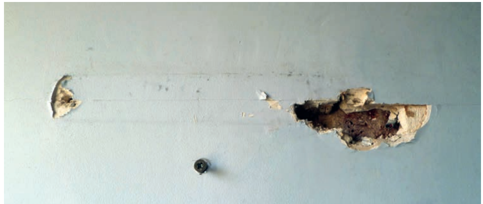
▲ Figure 4.10 Holes or cracks in walls
