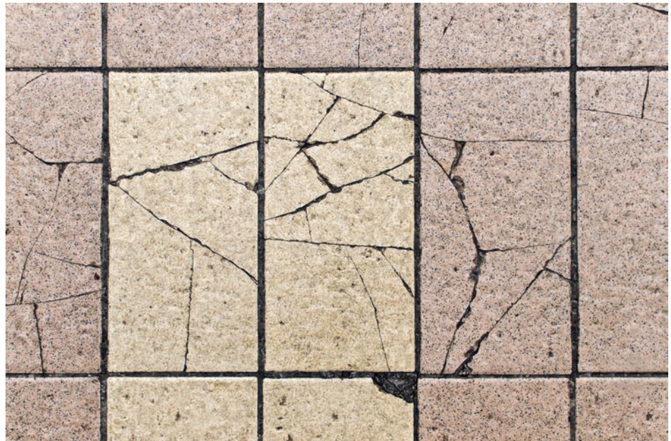
▲ Figure 4.17 Damaged wall tiles
