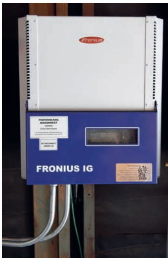
▲ Figure 1.27 Photovoltaic inverter
