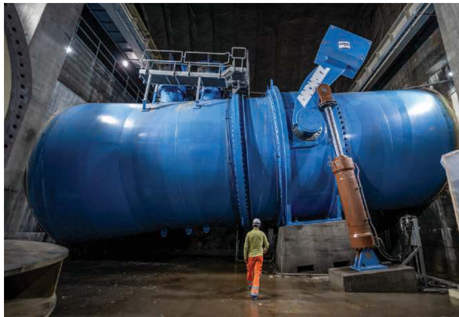
A massive penstock carries water between two reservoirs at Nant de Drance, a 900-megawatt plant in Switzerland.
