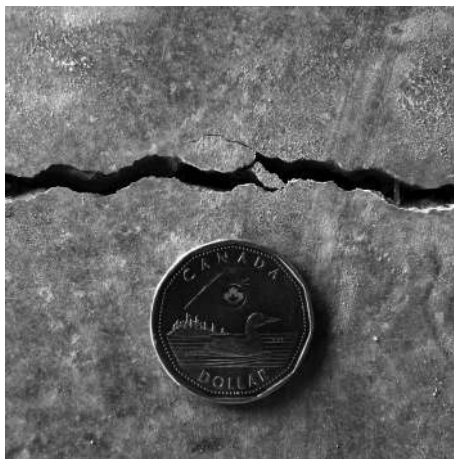
FIGURE 13.5 An uncontrolled drying-shrinkage crack. Few users will accept a crack like this. The coin has a diameter of 26.5 mm.
