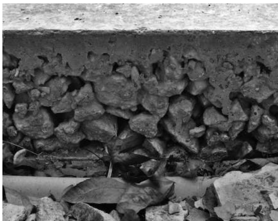
FIGURE 10.7 This concrete was not compacted.
