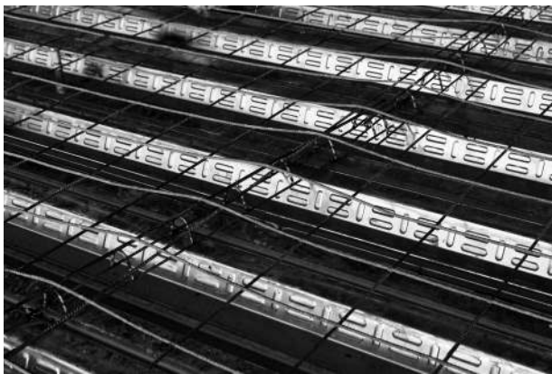
FIGURE 12.2 Wire mesh in a composite slab. Note the sagging caused by excessive distance between supports.
