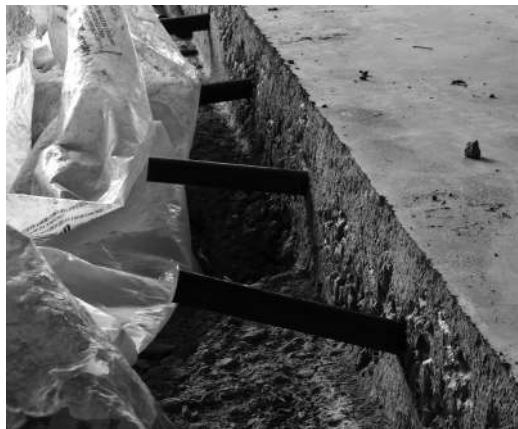
FIGURE 15.5 Dowels should be perpendicular to the plane of the joint so the joint can open and close. These crooked dowels might as well be tie bars.
