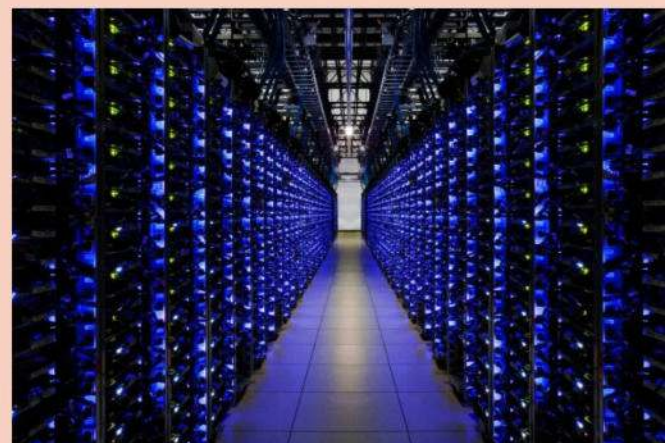
Rows upon rows of servers all work together to form the Google AI Cloud.
