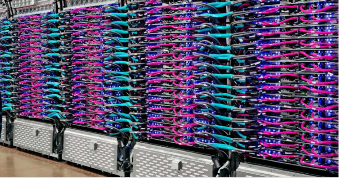
A slice of one of the many Google AI Cloud Data Centres cooling solutions.
