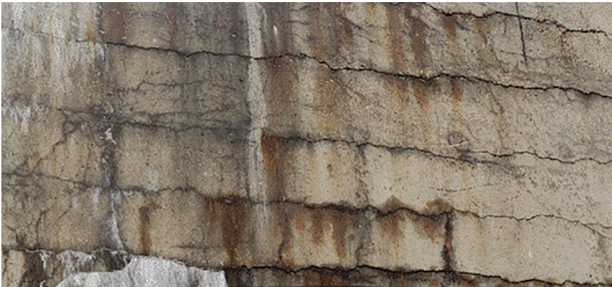
FIGURE 1.1 Degradation of concrete structures due to the influence of aggressive chemicals.
