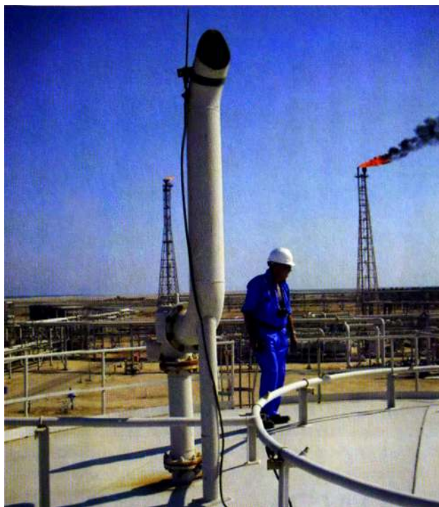
Figure 23.77 Vent from a hydrocarbon condensate tank with lightning conductor.
