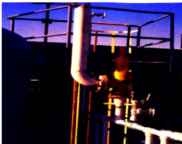
Figure 23.20g Inlet piping expanding into the relief valve. Incorrect installation may lead to valves chattering. (Source: Chris Flower and Adam Wills, The Chemical Engineer, U.K., pp. 24-31, June 2017.)
