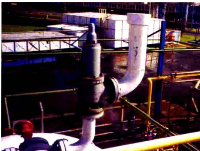
Figure 23.20h An unrestrained metal cover placed over an outlet pipe could become a missile. (Source: Chris Flower and Adam Wills, The Chemical Engineer , U.K., pp. 24-31, June 2017).
