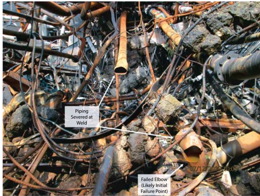
Figure 24.23 Photo of ruptured pipe elbow found post-incident (www.csb.gov).
