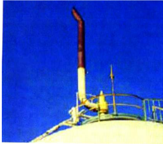
Figure 23.75 Unsupported discharge pipework – reaction forces are likely to cause damage to the relief valve and vessel nozzle.
