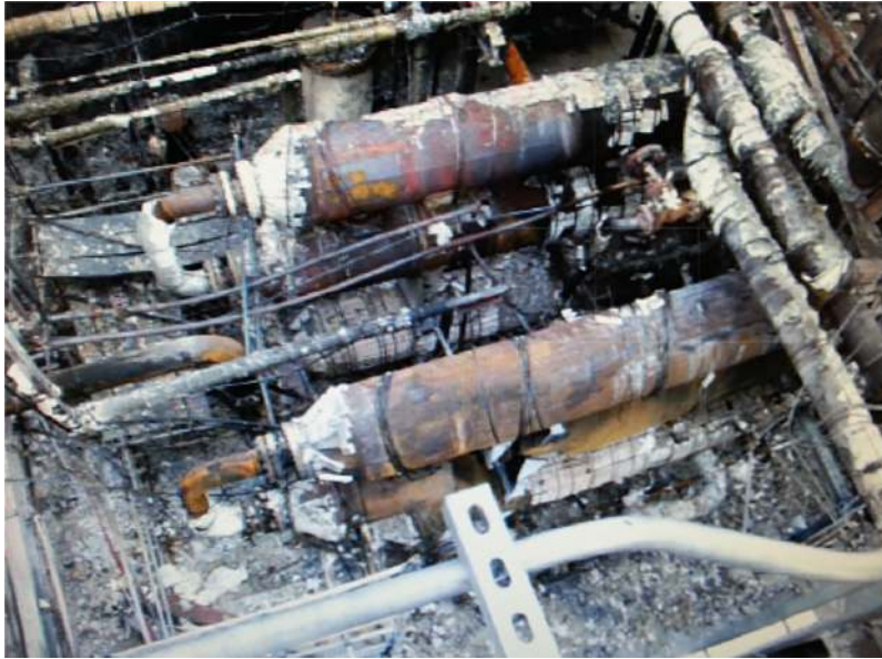
Figure 24.13 Aerial view of the damaged heat exchangers at Tesoro Refinery in Washington, DC (Source: www.csb.gov).
