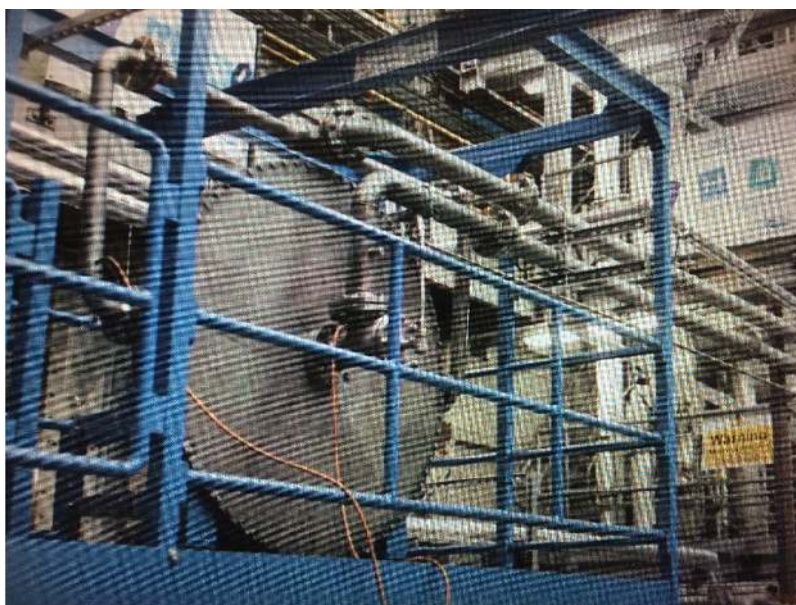
Figure 27.79 Large scale of CycloneCC (Source: Carbon Clean Solution Ltd.).
