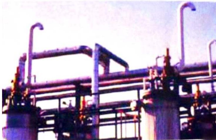
Figure 23.76 Long unsupported relief discharge lines are likely to fail in a relief vent.
