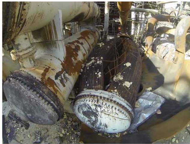
Figure 23.84 Post – incident photo of the ruptured Reboiler B. (Source: www.csb.gov).
