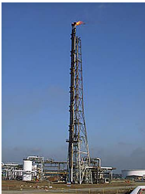
Figure 24.44 Flare stack at the Shell Haven refinery in U.K. (Source: www.en.m.wikipedia.org ).
