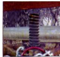
Blockage found in Valve "C" and close up of valve stem showing that it was not fully closed
