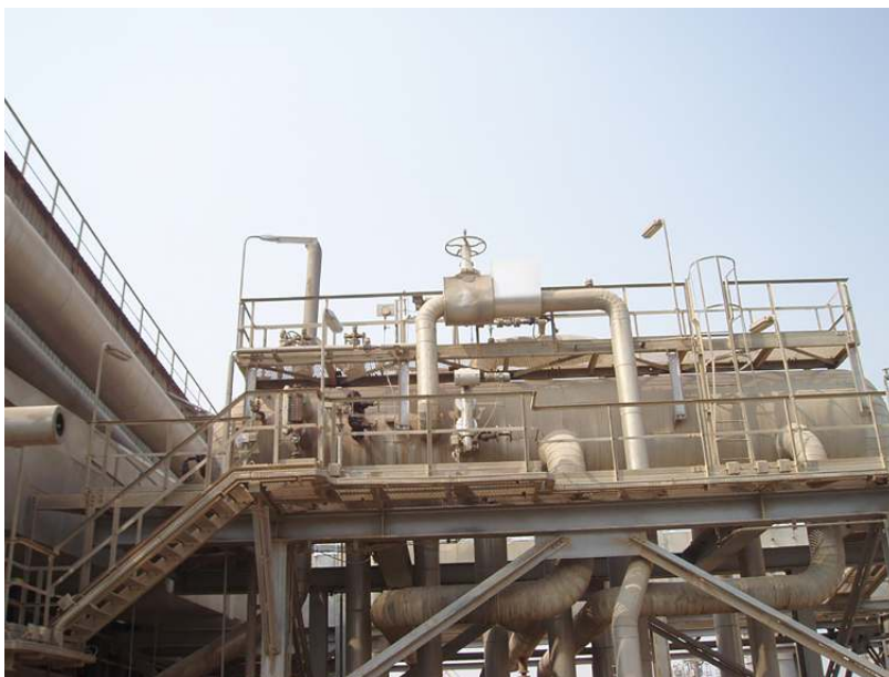
Figure 18.55 A photograph of a horizontal separator in a refinery facility.
