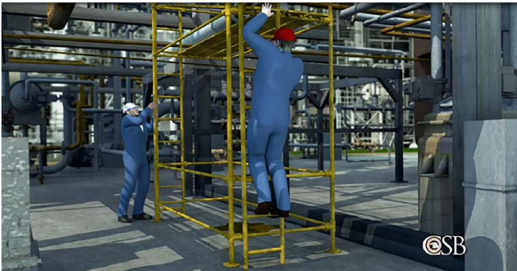
Figure 19.212 CSB animation of contractors erecting scaffolding beneath the leak location (Source: www.csb.gov ).
