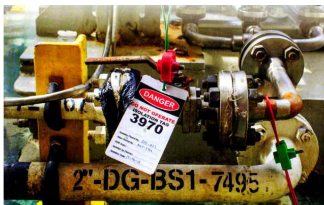
Figure 25 An isolation tag on a piece of equipment (Source: hazarddex, www.hazardexonthenet.net).
