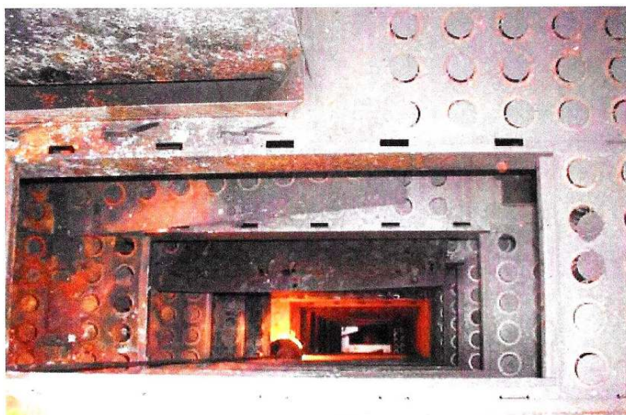
Figure 19.143 Gasoline splitter - installation problem of the column. Column suddenly lost all separation.
