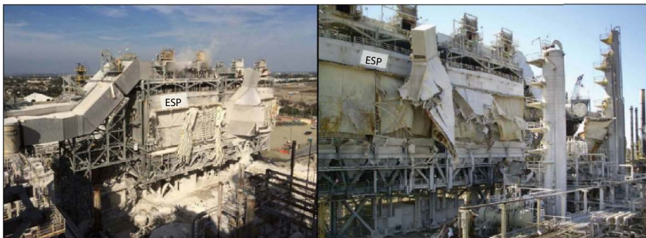
Figure 18.148 Damage to the ESP from the explosion. White catalyst dust from the ESP is visible on the ground in left photo (source: www.csb.gov).
