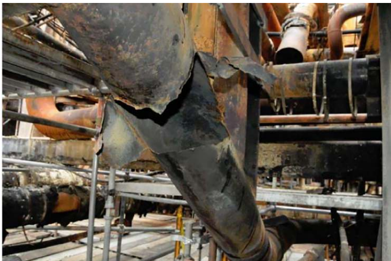
Figure 19.209 Photo of rupture on 4-sidecut 52-in. component (Source: www.csb.gov).
