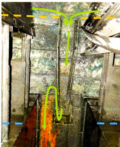
Figure 19.152 Tray downcomer connection and the flow path (Source: Ozturk, G., et al. Hydrocarbon Processing, Feb. 2021 [237]).
