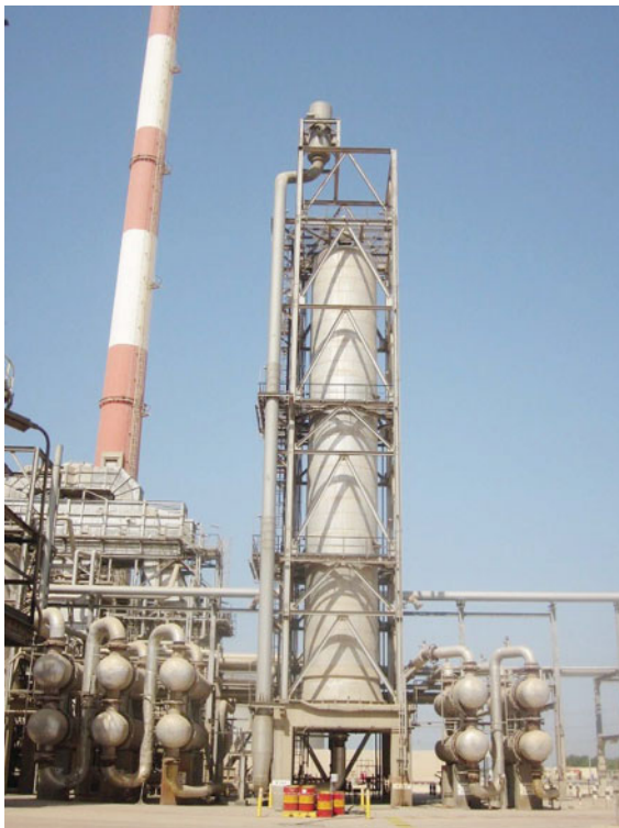
Figure 7.40 Heavy gas oil hydrodesulfurizer reactor with feed/effluent shell and tube heat exchangers.
