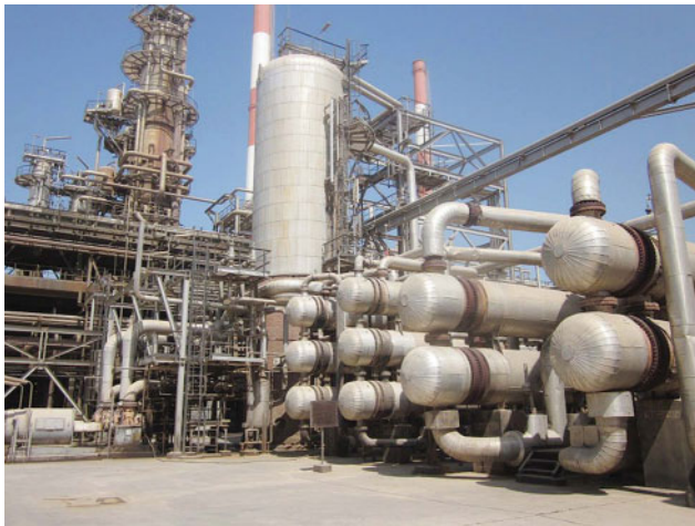
Figure 5.13 A photograph showing the crude distillation column, a pre-flash vessel and pre-heater shell and tube heat exchangers in series.
