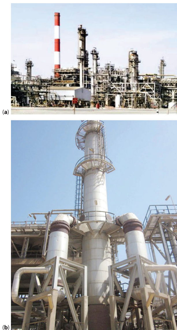
Figure 5.7 (a) Photograph of a refinery with fractionating columns, associated piping and ancillary equipment. (b) Photograph of the naphtha stabilizer column equipped with two vertical reboilers in the crude distillation unit.
