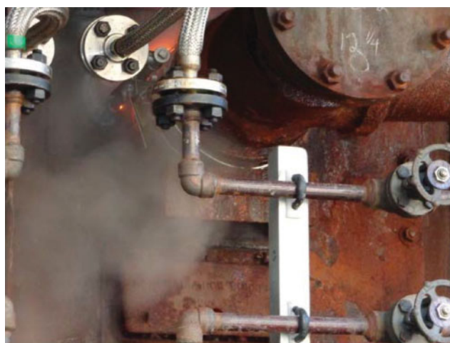
Figure 10.20 Burner on furnace (Source: csb.gov).
