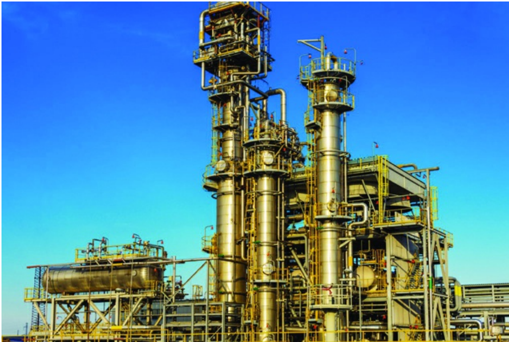
Figure 5.1 Section of a large ammonia plant showing the equipment in place (Image courtesy of nepper77/Shutterstock)
