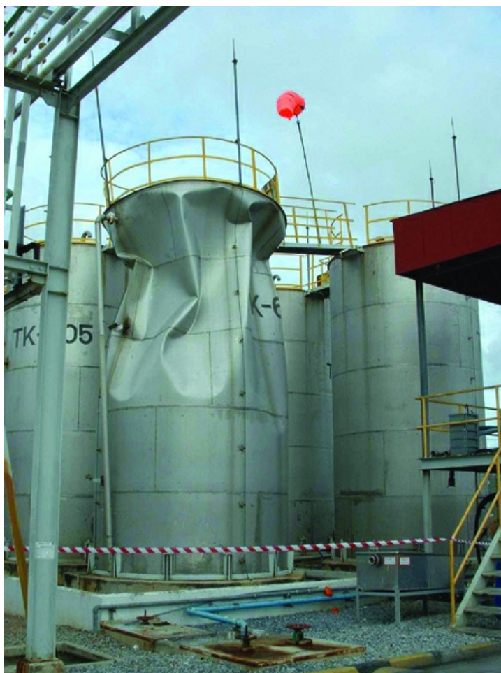
Figure 2.6 A failed tank. (Image courtesy of "CCPS Process Safety Beacon," AIChE)
