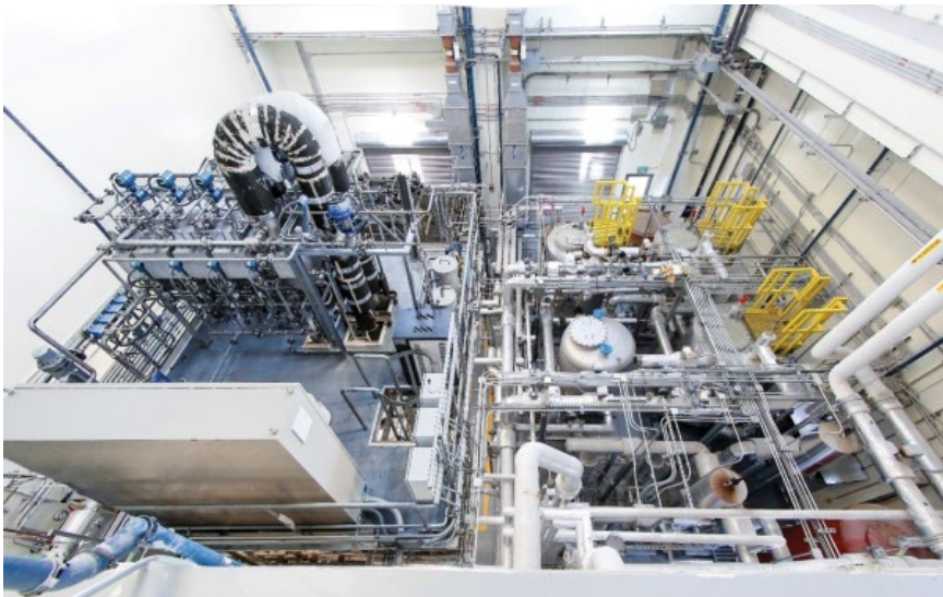
Figure 11.15 Pilot MEDAD hybrid plant installed at KAUST.
