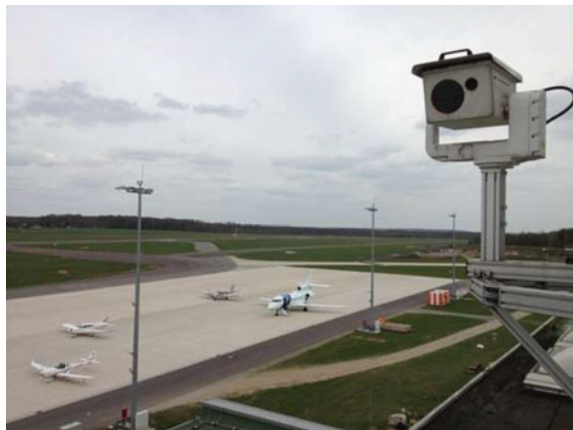
Fig. 10 FLIR thermal imager (large circular Ge-window) as part of the DLR-RTO system at Braunschweig airport, integrated in a remotely controlled housing together with visual PTZ camera
