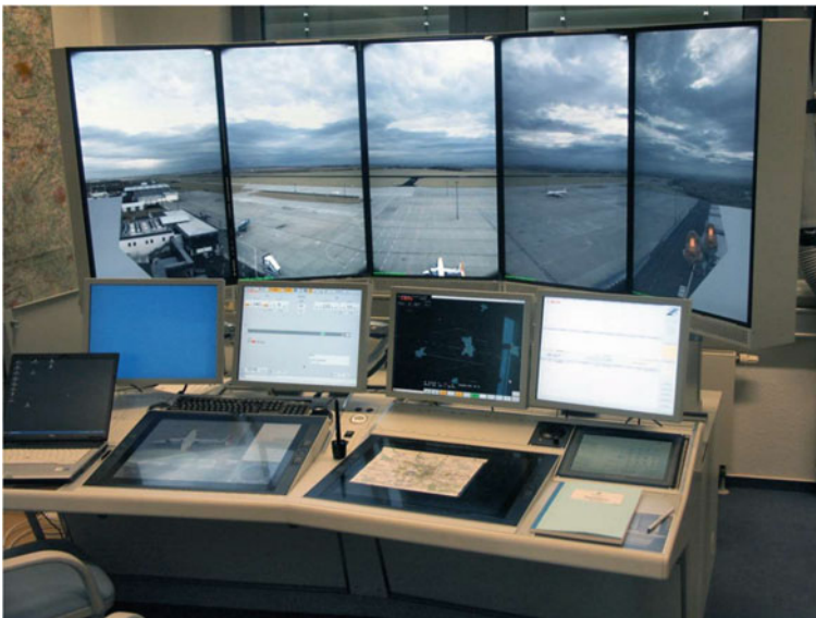
Fig. 4 Implementation of the R-CWP at Erfurt tower control room without direct airport view. Three levels of information with the video panorama in the back, the row of four flight information displays, operator console with two large touch-input displays and a small one at the right side for radio communication, are clearly structured (for details see text)
