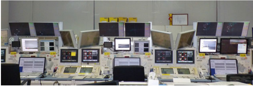
Fig. 2 Remote AFIS operation room in FSC
