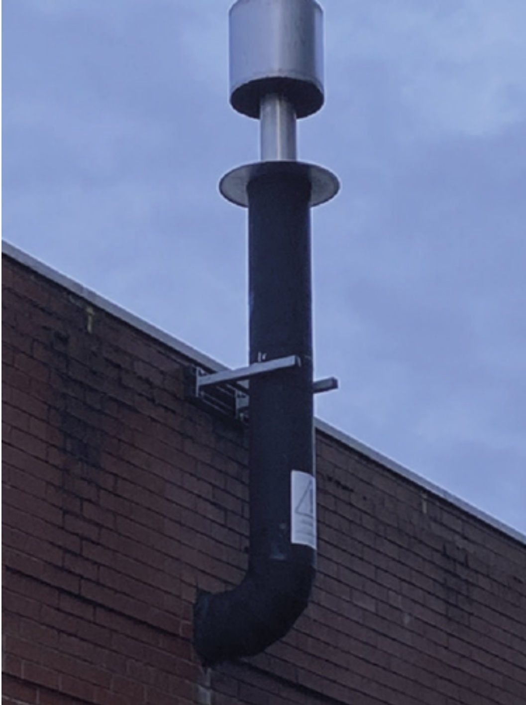
Fig. 1.7a External quench pipe. 📄
